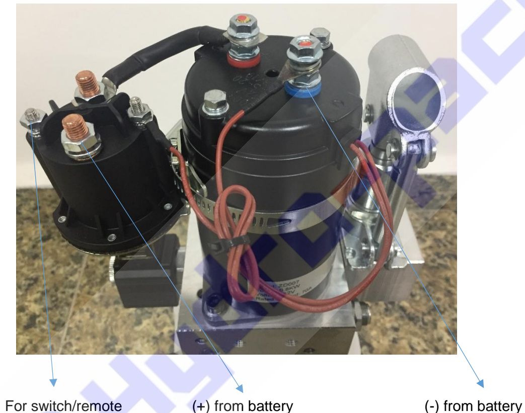
Photo 3. Connection on DC motor
